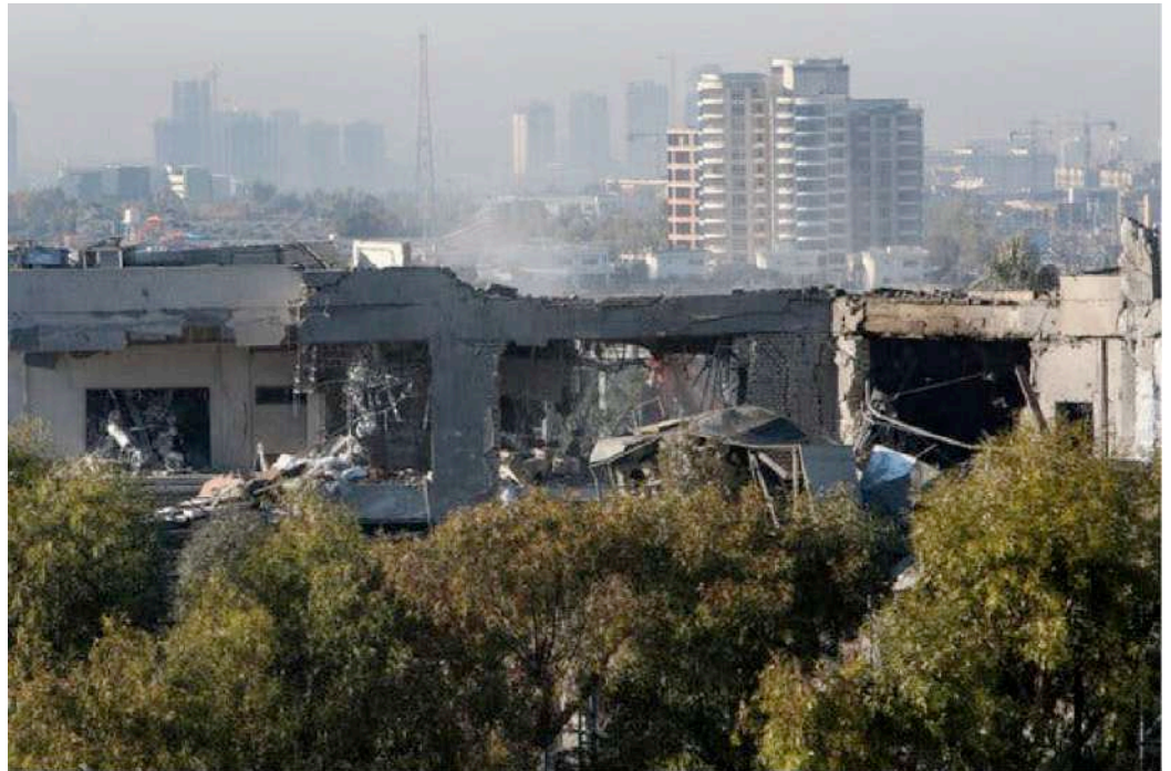
A damaged building after missile attacks in Erbil, Iraq, on Tuesday. Azad Lashkari/ Reuters
